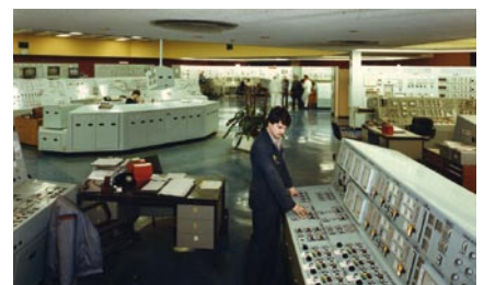
Original control room at Drax
